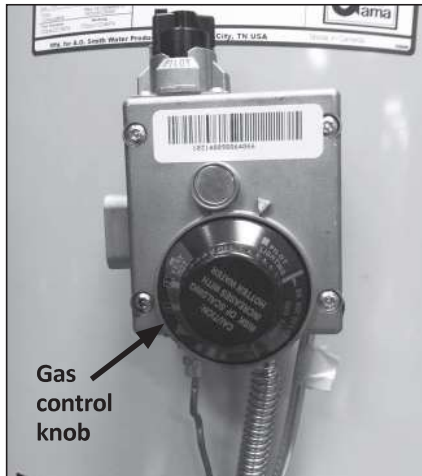
Figure 17 - Turn gas control/temperature knob OFF.
