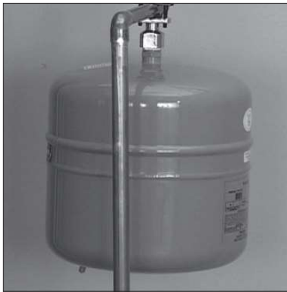
Figure 28 - The Thermal Expansion Tank should be pressurized with air, using a hand pump, to match the home's incoming water pressure.
